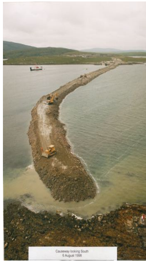
The causeway nears completion. The first crossing on foot was in August 1998.
